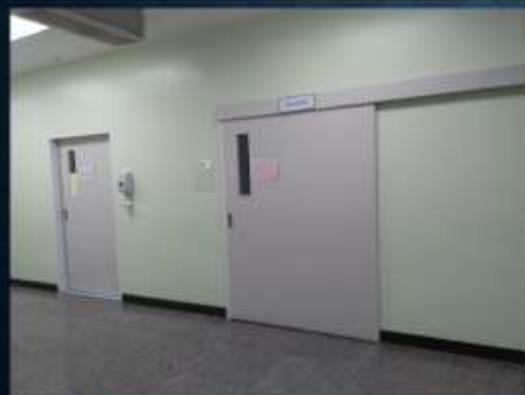
Negative pressure room
